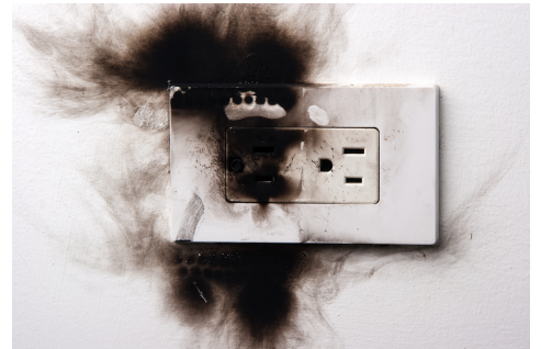
Scorch marks on cover plate
