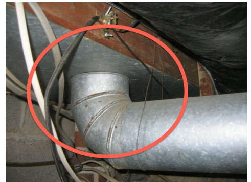
Loose connection; recommend sealing.
